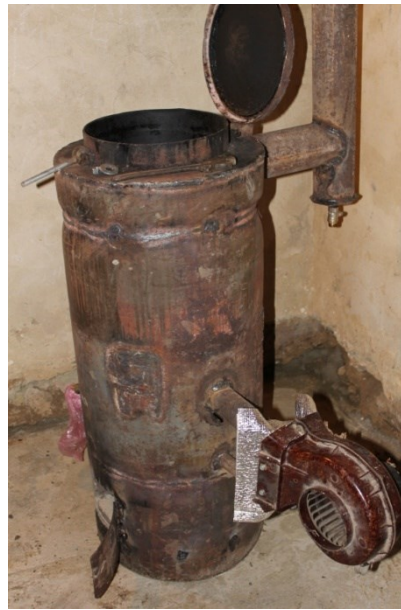
Fig. 4.12 Pilot of gas-fired boiler
