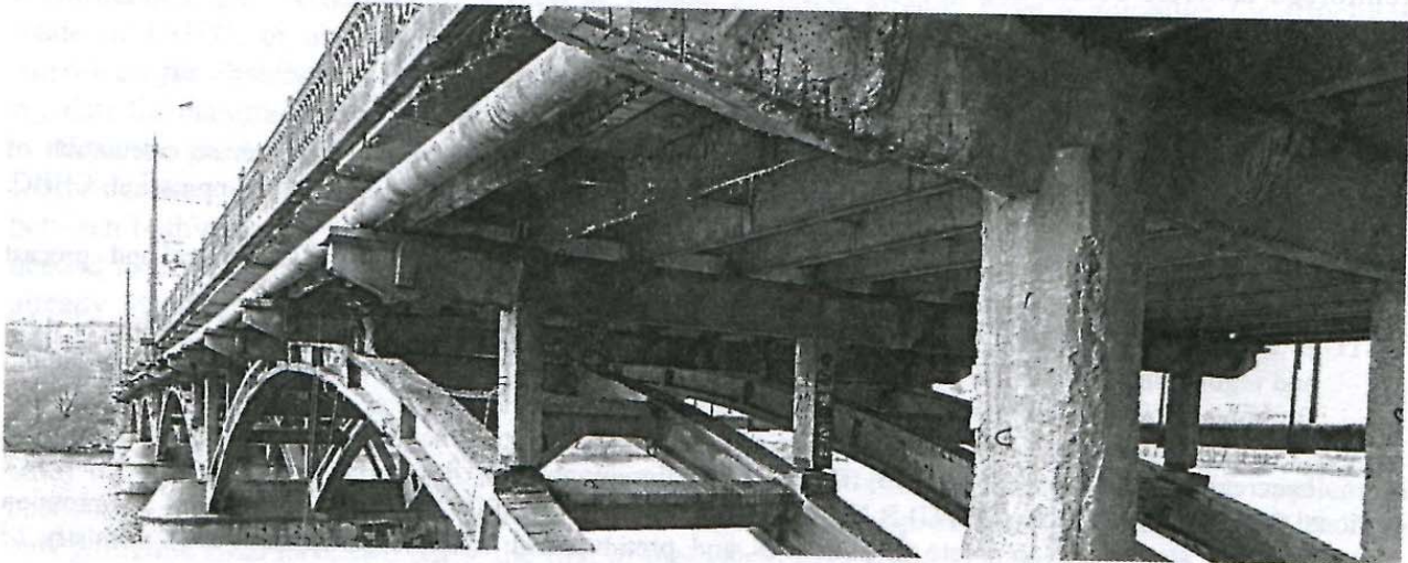
Figure 1. The general condition of the arched span structure of the bridge in Chornovol street before the reconstruction.
