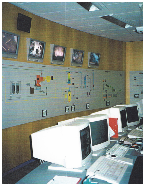
Figure 6.8. Control center of waste incinerator
