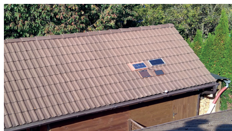
Fig. 1. View of the model installation
