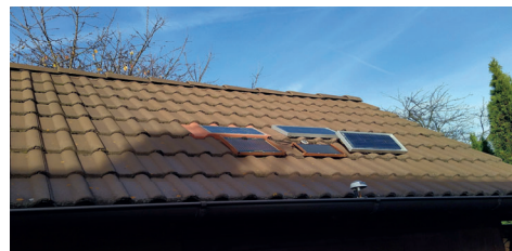
Fig. 8. Shading of the panels by the passing shadow of the chimney
