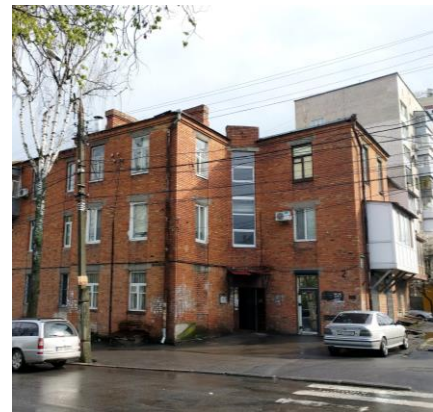
Fig. 4. Residential house on 2 Vladyslav Gorodetskiy St., 5 Lev Tolstoy St., Vinnytsia (© Subin-Kozhevnikova A. S., 2017)
