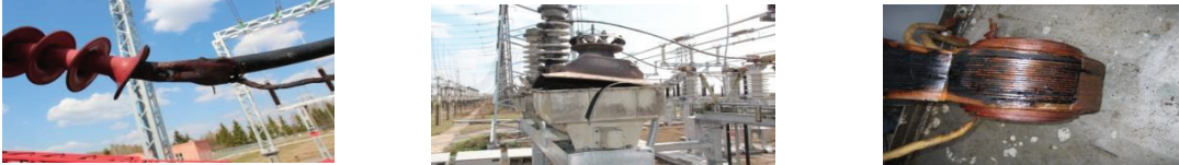
FIGURE 3. Examples of damaged high-voltage equipment and paper insulation
