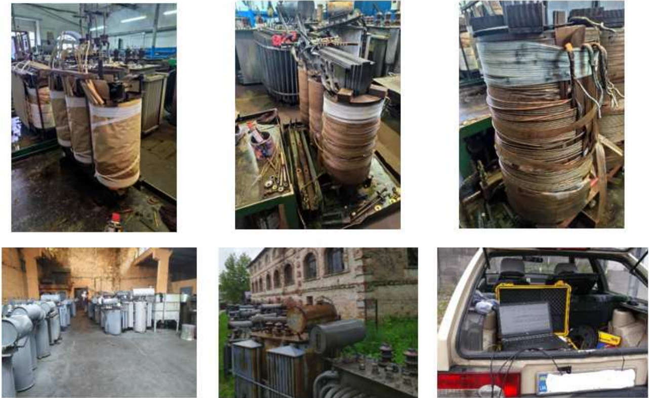
Fig. 2. Damaged and repaired power transformers of 10 kV section of repair of PTs power supply company (Vinnytsiaoblenergo).
