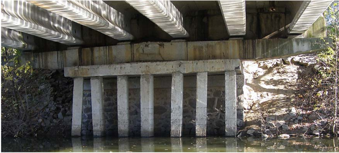
Figure 1 – Example of a typical crossbar system (constant height) of a beam bridge, where the pile foundations perform the function of the shaft of the bridge abutment
