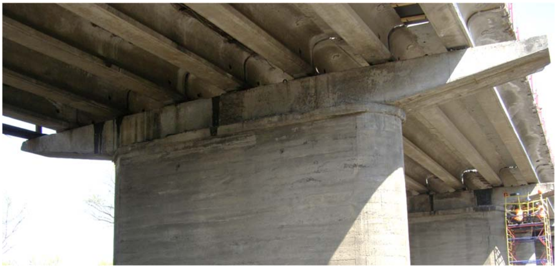
Figure 2 – Example of a typical crossbar system (variable height) of a beam bridge, where the central trunk of the bridge support is made in the form of a massive rod
